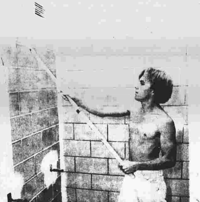
Work crew member Carl Gaylor puts a coat of fresh white paint over a dingy blue wall in the girls' locker room.
